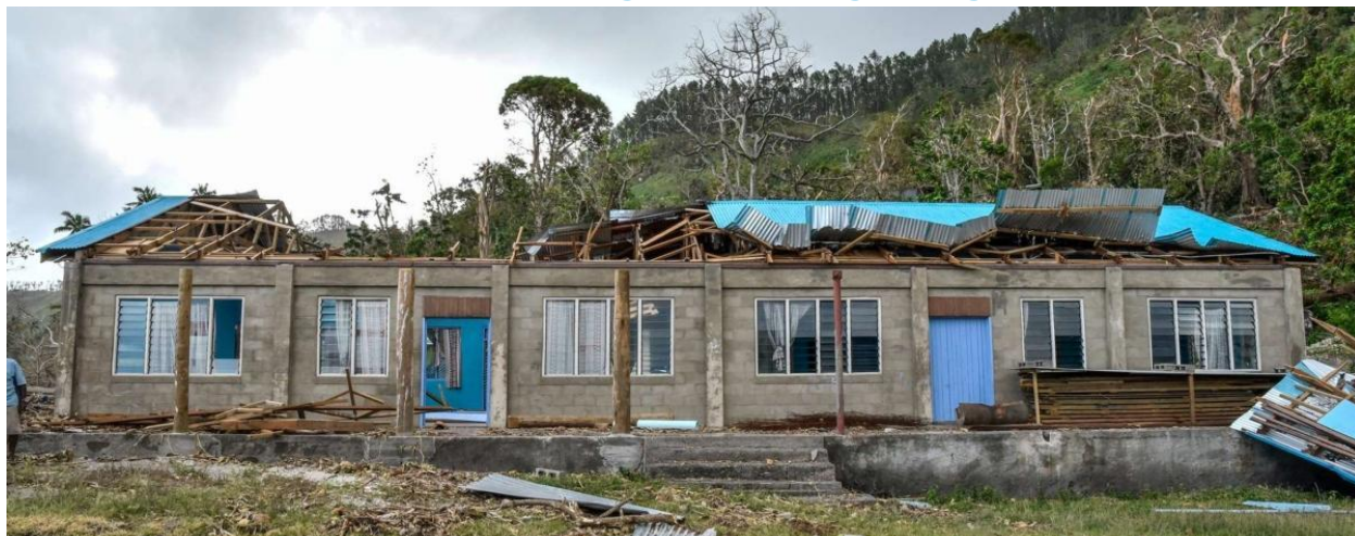
Damaged Dagai village hall in Kadavu, Fiji | © Fiji Climate Change Portal
